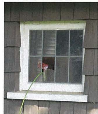
Broken window pane on south elevation
