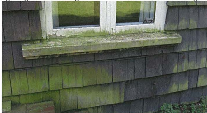
North elevation window frame and sill showing deterioration
