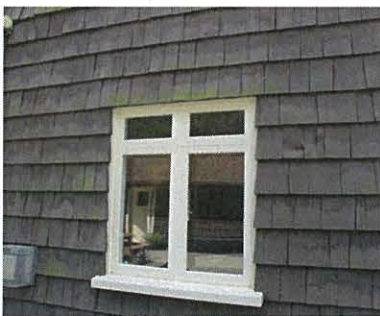
Wavy water damage visible
