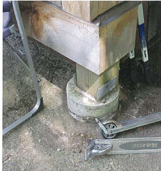
Void where brick steps should be extended
