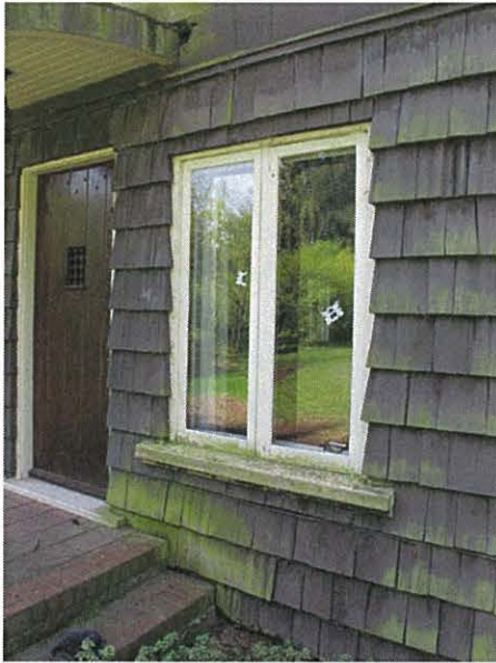
North elevation: biological growth on shingles
