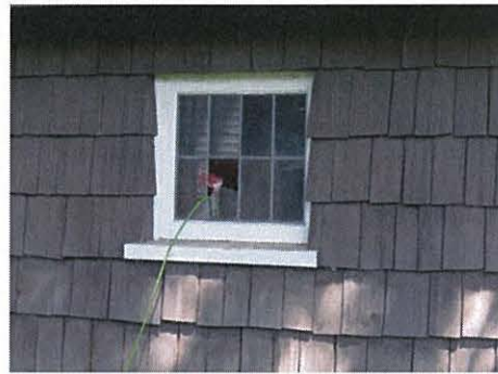
Example: window (broken pane)
