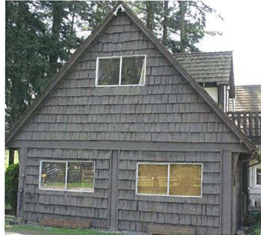
Non-original metal windows on the northeastern elevation, which should be replaced with more historically appropriate wooden frames and sashes
