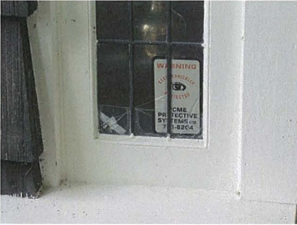
Close-up of the broken glass of the sidelight of the front door
