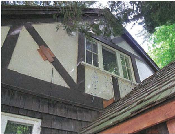
South elevation: half-timbering (to be repaired), wood trim and projected sill
