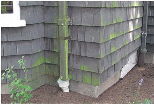
Biological growth on exterior walls (see the last bullet point of this section on page 18)
