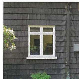
Damage by drainpipe visible
