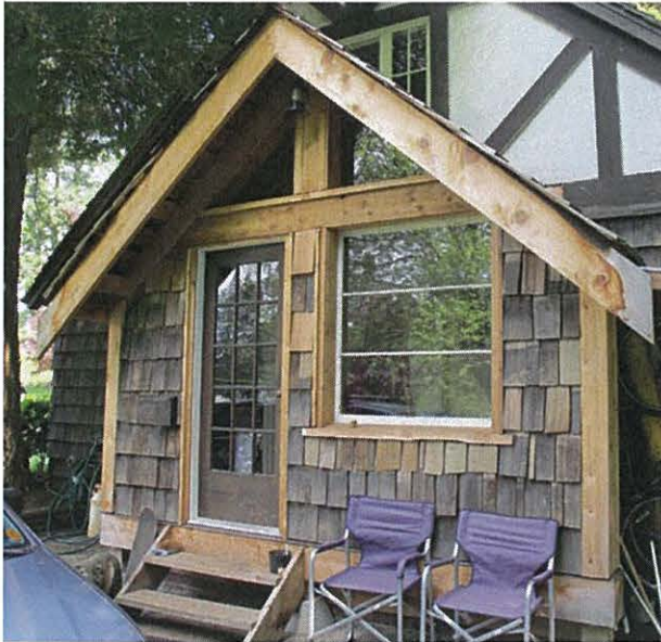
South elevation entryway addition: door, window, bargeboards, cornerboards and shingles should more closely match the remainder of the cottage
