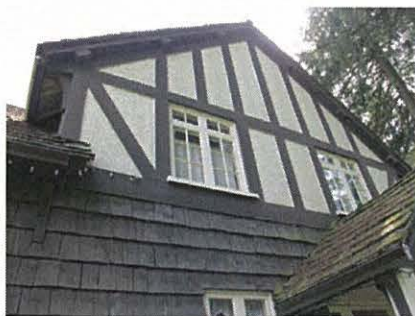
Wavy water damage visibly
