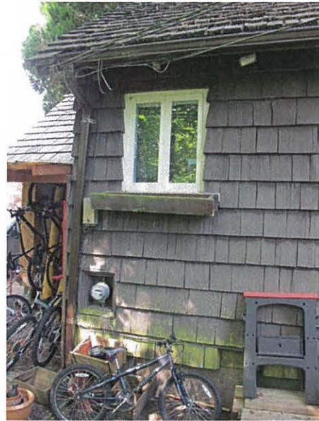
East elevation: biological growth on shingles
