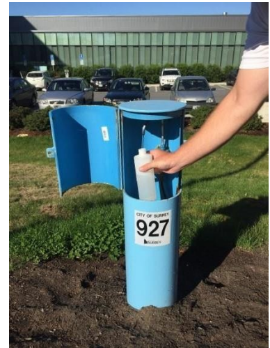
Water Sampling Station at 148
